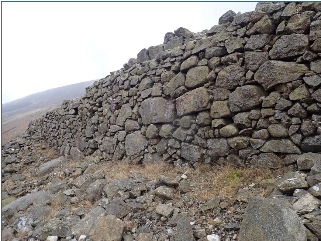
Figure 21 Retaining wall of buddle amongst which patches of Cephaloziella cf. nicholsonii grow.
