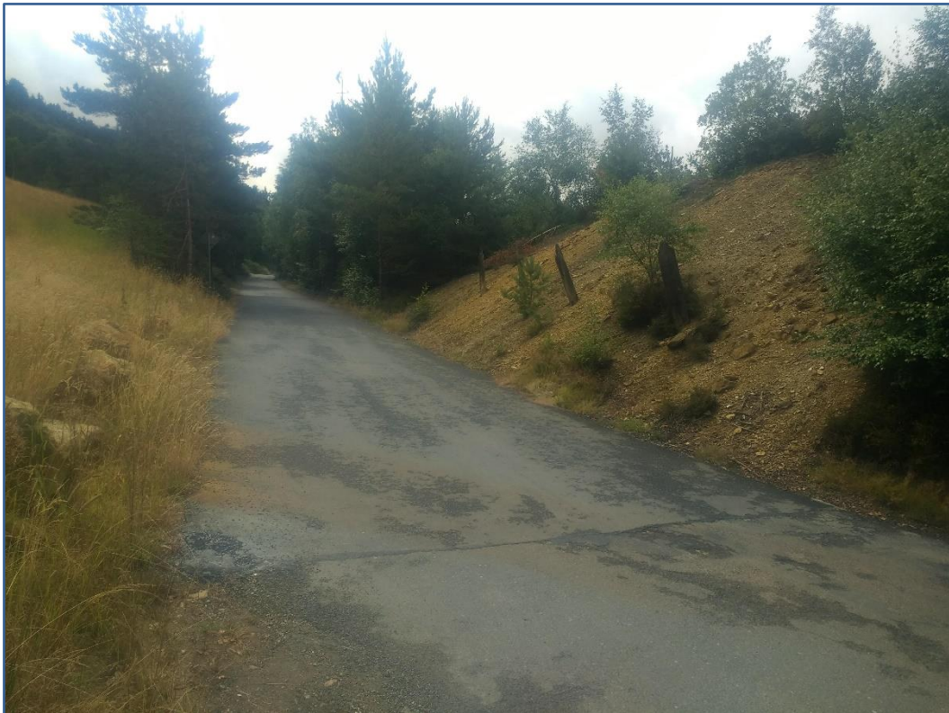
Figure 42 Bare spoil remaining between minor road and the railway, with small patches of Calaminarian grassland vegetation present.
