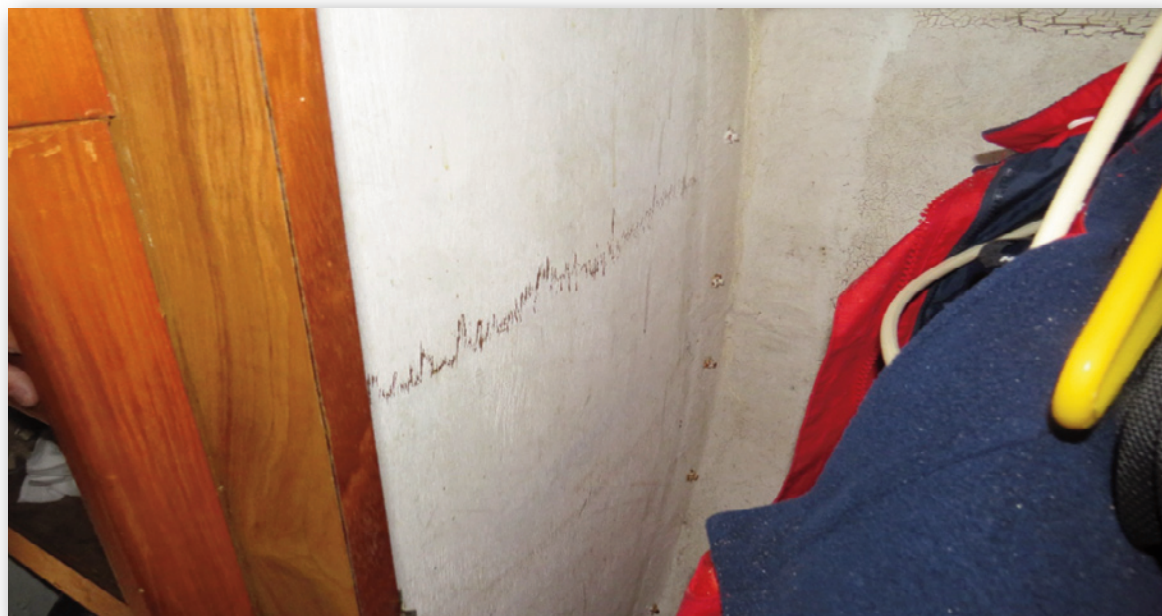
Photograph No.6 - Internal damage to bulhead.
