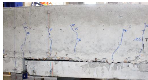
Figure 10: 400 mm of delamination.
