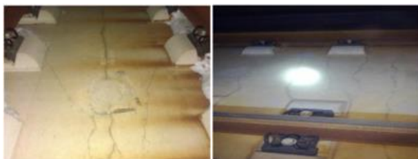
Figure 1: Cracking of CRTS type III track plate on the bridge
