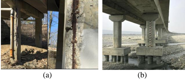
Figure 1. Illustration of study object: (a) typical corrosion issues for bridges (photo by the authors), and (b) a typical highway bridge in a scour scenario (by courtesy of Professor Yi-Ching Lin)
