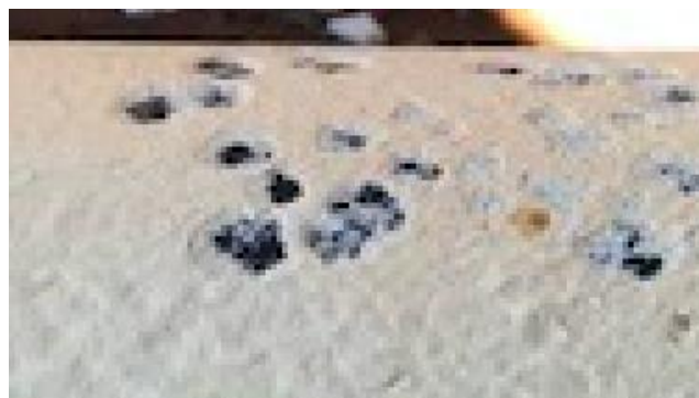
Figure 1: Local failures of protective coating.
