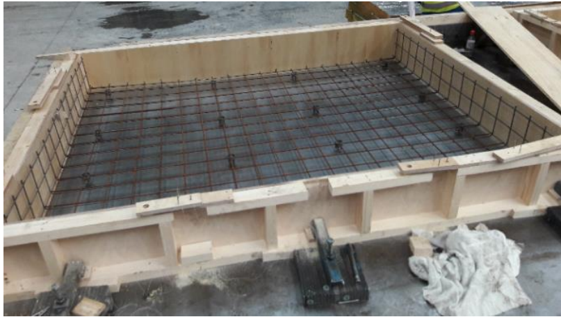
Figure 7-6 Steel mesh reinforcement for the 70 mm concrete outer leaf was fixed into the formwork.
