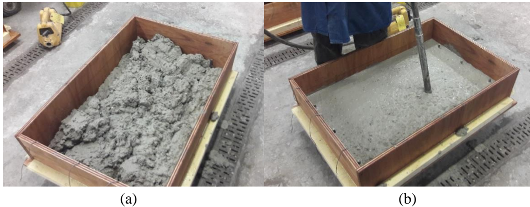
Figure 5-5 (a) Placement of the PCM-concrete composite in the formwork and (b) Compaction of PCM-concrete with a poker vibrator
