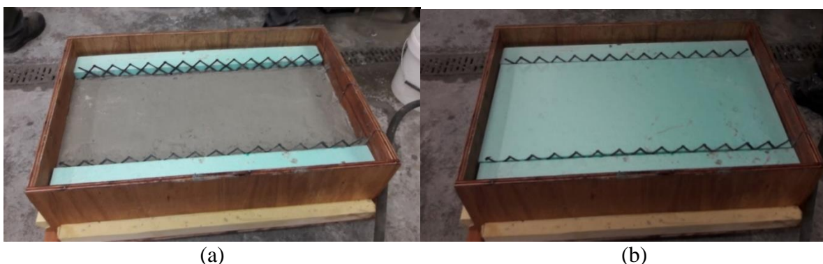
Figure 5-6 (a) Positioning of C-Grid connectors and (b) Insulation in place showing protrusion of C-Grid above the insulation
