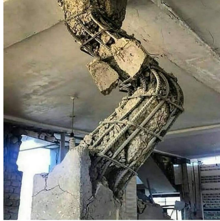
Figure 1.2: A disturbing sight at a construction site! The critical load on this steel-reinforced concrete column has been exceeded, and caused the column to buckle (the lateral displacement of the steel frame). This is unlikely to be elastic buckling, i.e. the steel will not return to its original shape when the weight is removed, but it does show the expected profile of a buckling beam. Image taken from https://www.pinterest.com/CivilEngDis/ .
