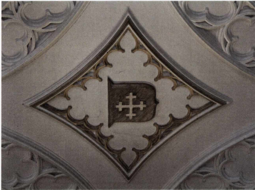
Fig. 3.100 Charleville Castle, detail of fan vaulting, gallery, showing Bury coat of arms, Francis Johnston, modelled c.1807-8, photograph Judith
