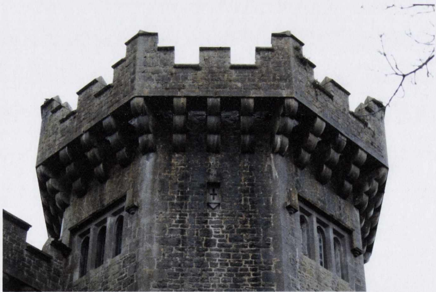
Fig. 3.75 Charleville Castle, north elevation, detail of corbelling on octagonal tower, Francis Johnston, constructed 1801–1804, photograph Judith Hill, 2016.
