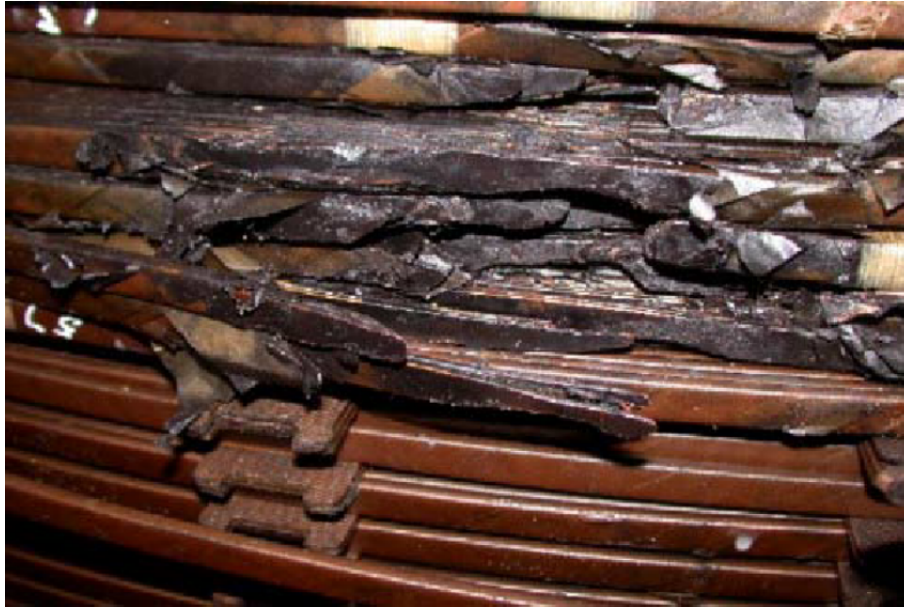
Figure 1.6: Failure in a transformer three weeks following the Halloween storm, 2003, in South Africa (Thomson et al., 2010). Damage sustained from the storm led to overheating in the transformer, later leading to an arcing fault (an electrical fire).
