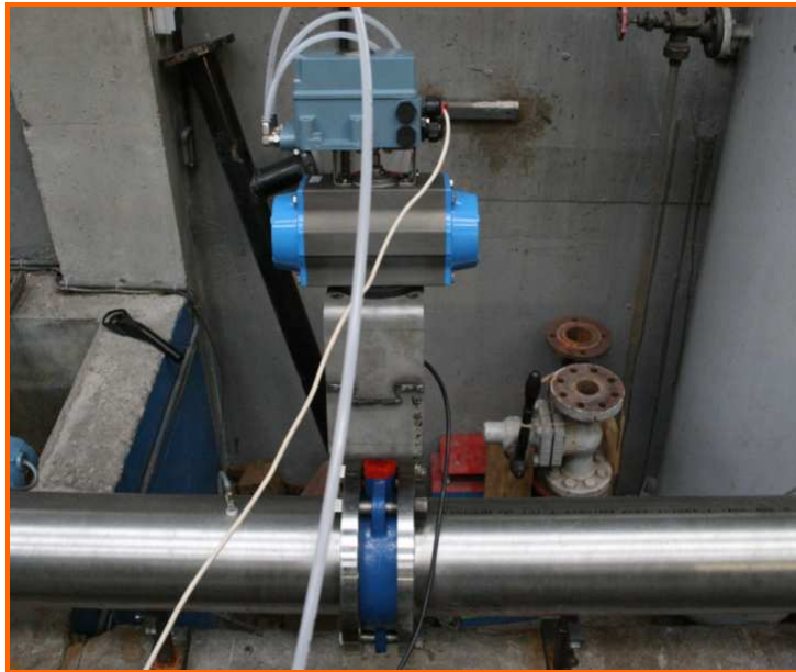
Figure 3.14 : The torque-meter above the butterfly valve
