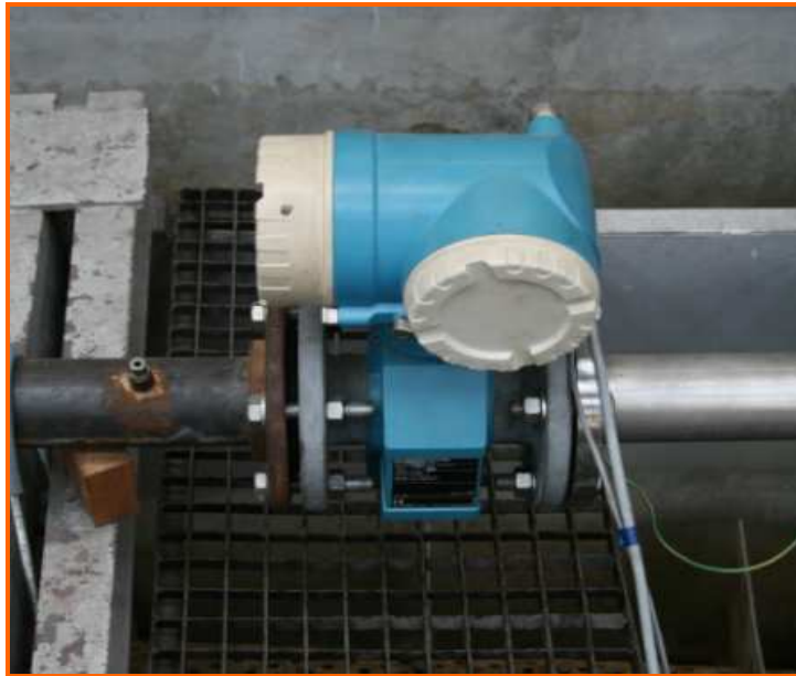
Figure 3.12 : The flow rate meter at 14 D upstream from butterfly valve
