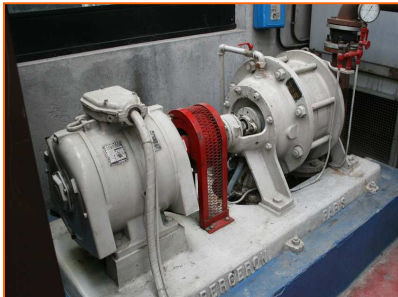
Figure 3.9 : The 14.7 KW centrifugal water pump
