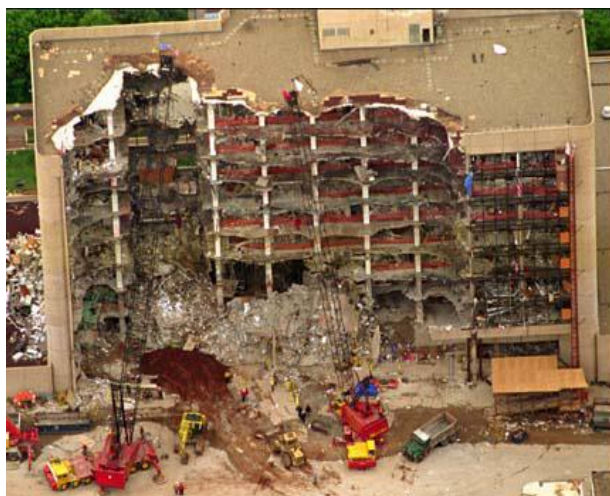
Figure 2.8 Damage to the Murrah Building, as a result of the blast and the subsequent progressive collapse
