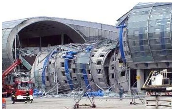
Figure 2.17 Partial collapse of Charles de Gaulle Airport Terminal 2E
