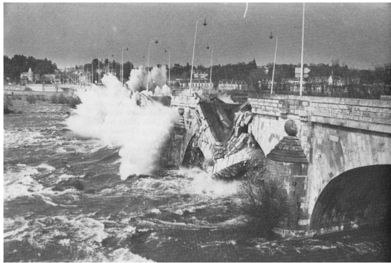
Figure 1.1 Progressive collapse of masonry arch bridge over the River Loire (Heyman, 1982)
