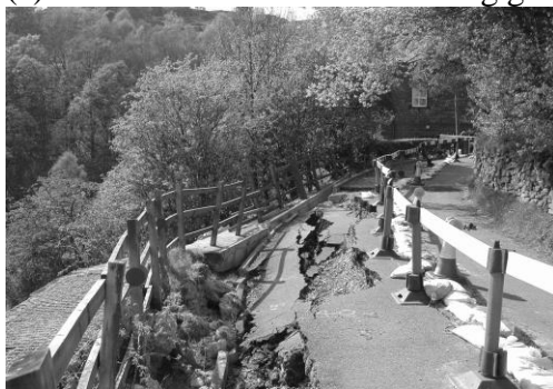
(c) Collapse of southern part of road.
