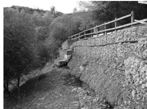
(b) Settlement of gabion wall foundations.
