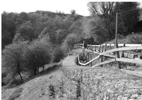
(a) Outward movement of existing gabion wall.
