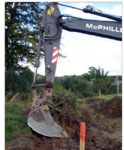
Figure 3. Placing a hedge section in the receptor trench, which had a slow-release fertiliser and water-retaining gel
