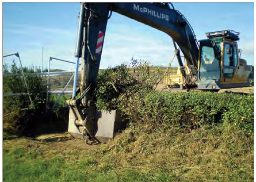
Figure 1. Mature hedges, which provide landscape structure, visual screening and wildlife corridors, can be excavated and moved to a new location rather than being cut down and chipped
