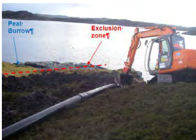
Photo 2. Case study 3 - works on a remote peninsula of the Isle of Lewis
