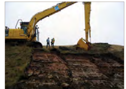
Figure 6. Removing 1 × 0.5 × 0.3 m turfs from the Boston Spa site with a modified bale-cutting bucket in spring 2006
