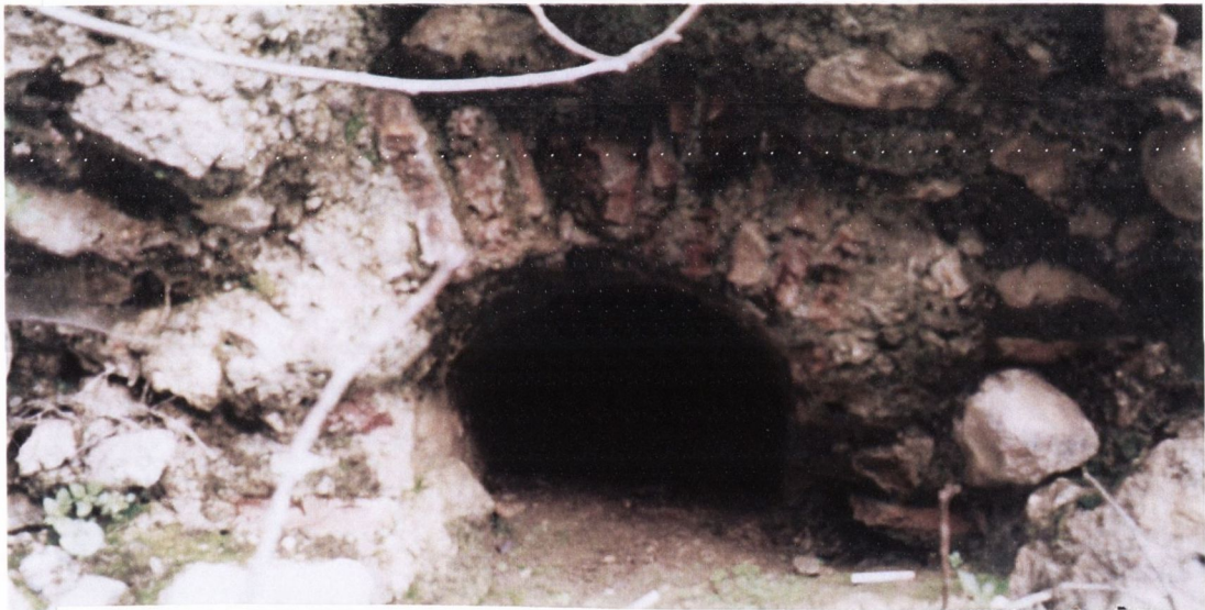
B Detail of drainage culvert in elevation extending south of caput aquae at Zaros
