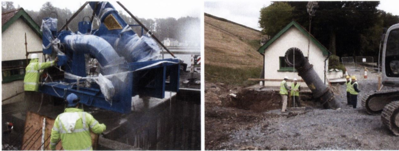
Fig. 7.5: Vartry waterworks turbine installation (L); Turbine intake (R).
