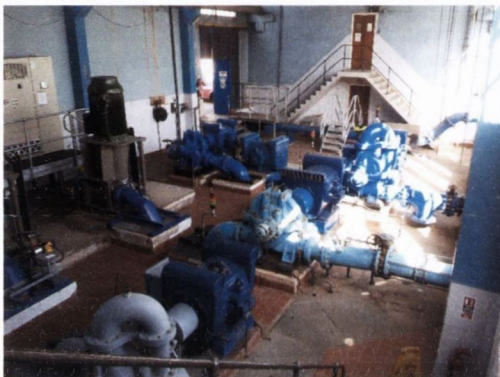
(c) Cork city water supply - pumping station
