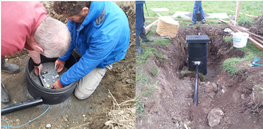
Figure 3.7: The Birr permanent magnetometer installation. Left: the plinth set in concrete upon which the magnetometer sits. Right: the inspection chamber before being buried. The thermal insulation can be seen on the left beside the trench.
