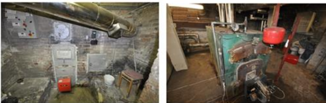
Figure 4.30 - Boiler room in Enniskillen (left) and boiler room in Killarney (right)
