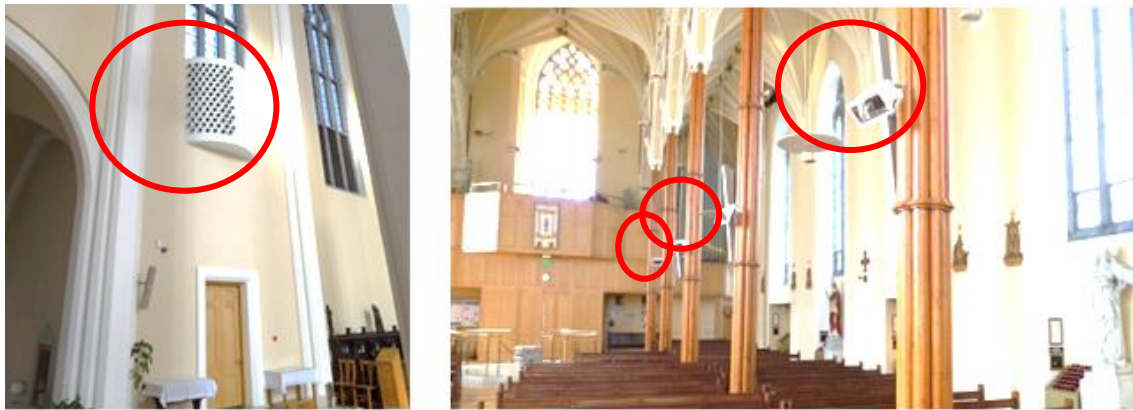
Figure 5.54 - Hot air blower outlet (left) and Electric radiant heaters (right) in St. Mary's Cathedral, Cork
