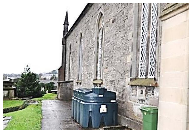
Figure 4.28 - Oil storage tank beside Enniskillen cathedral
