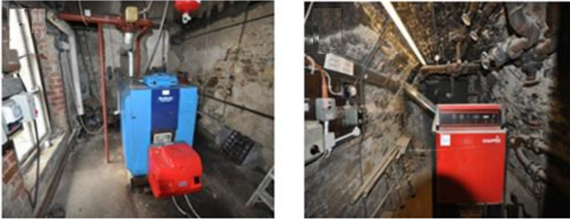
Figure 4.29 - Enniscorthy's boiler room and the boiler room in Down Cathedral where the names of the boilers are legible
