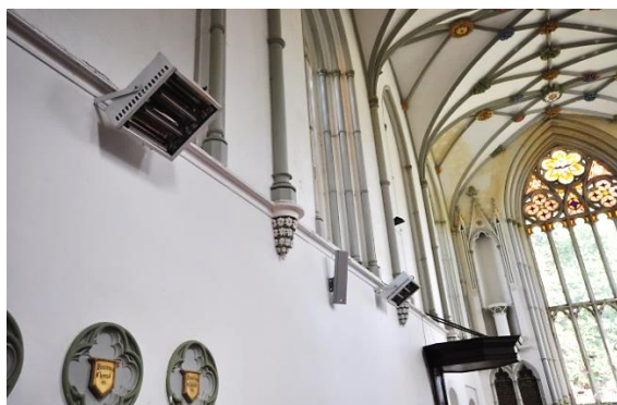
Figure 5.93 - The electric radiant heaters in Lismore Cathedral
