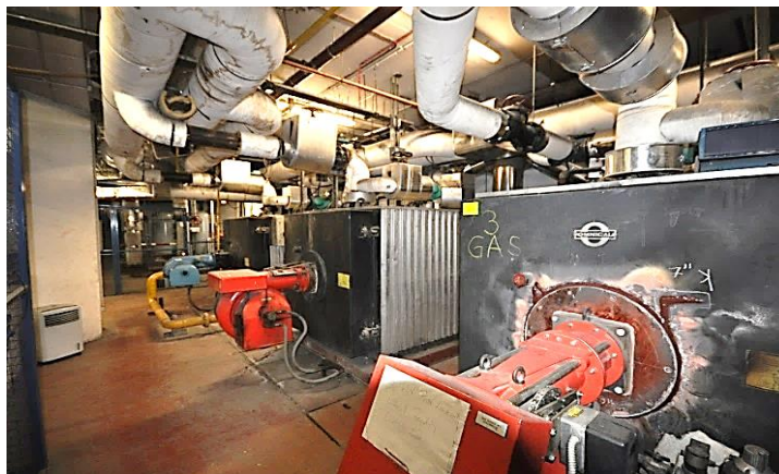
Figure 5.75 - Civic offices boilers which supplied heat to Christ Church cathedral, Dublin
