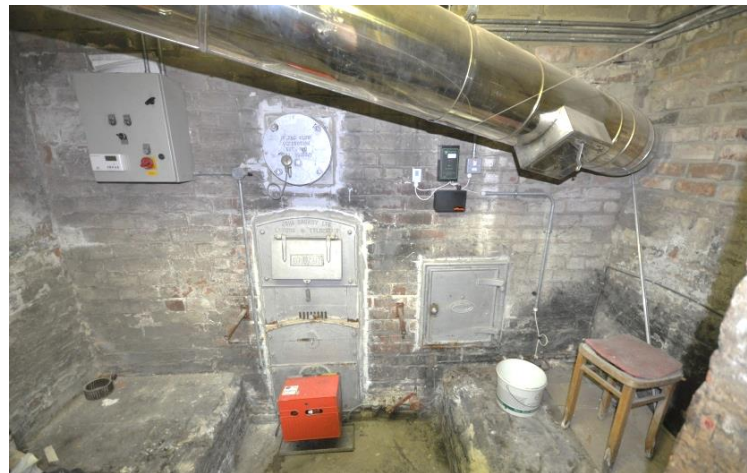
Figure 5.108 - Oil fired boiler in Enniskillen cathedral
