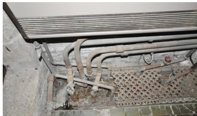
Figure 5.111 - Pipe work in St Brigid's cathedral, Kildare
