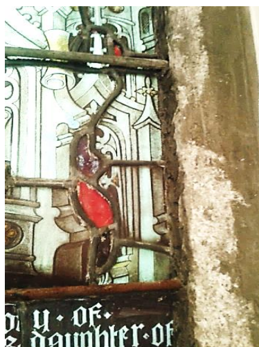
Figure 2.9 - A stained glass window, in an Irish church, showing salt damage near the tie bars
