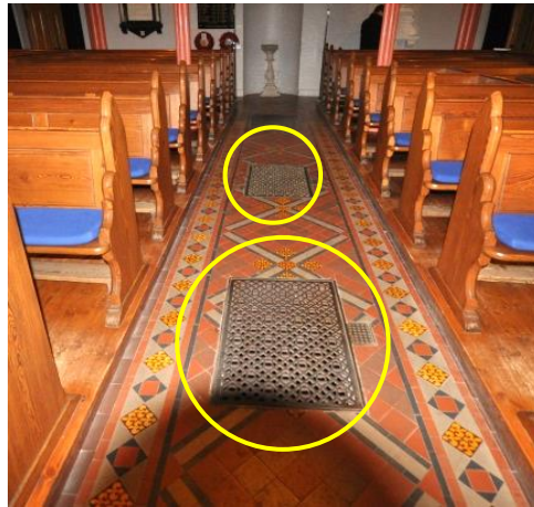
Figure 5.102 - Inlet and outlet grills for the hot air heating system in Enniskillen cathedral
