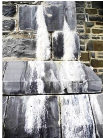
Figure 2.7 - Efflorescence on an East facing, outside wall of an Irish cathedral
