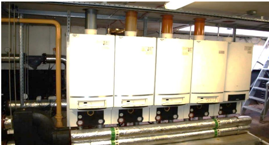
Figure 5.2 Gas boilers in St. Patrick's cathedral, Dublin
