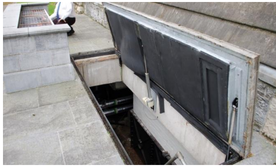
Figure 4.25 - Entrance to the boiler room of St. Patrick's cathedral, Dublin
