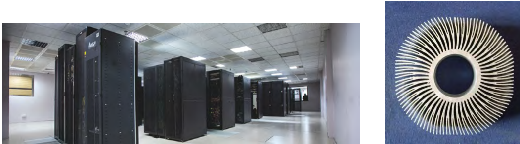
(a) Air-cooled data centre
