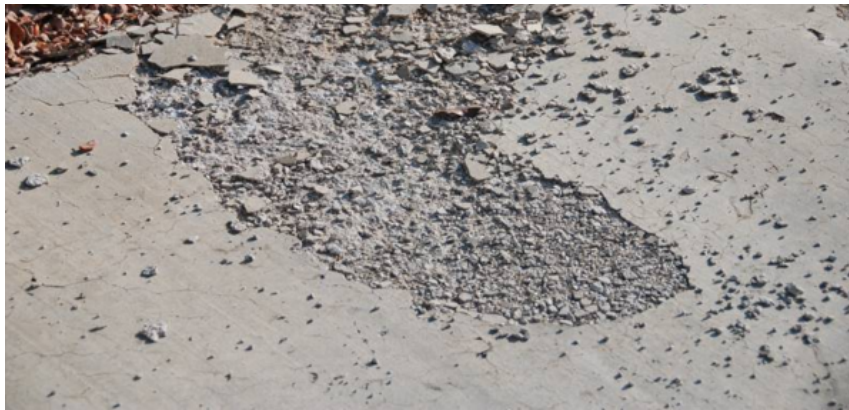
Figure 2.24: Spalling concrete: the loss of smaller amounts of materials from the surface is evident [137].
