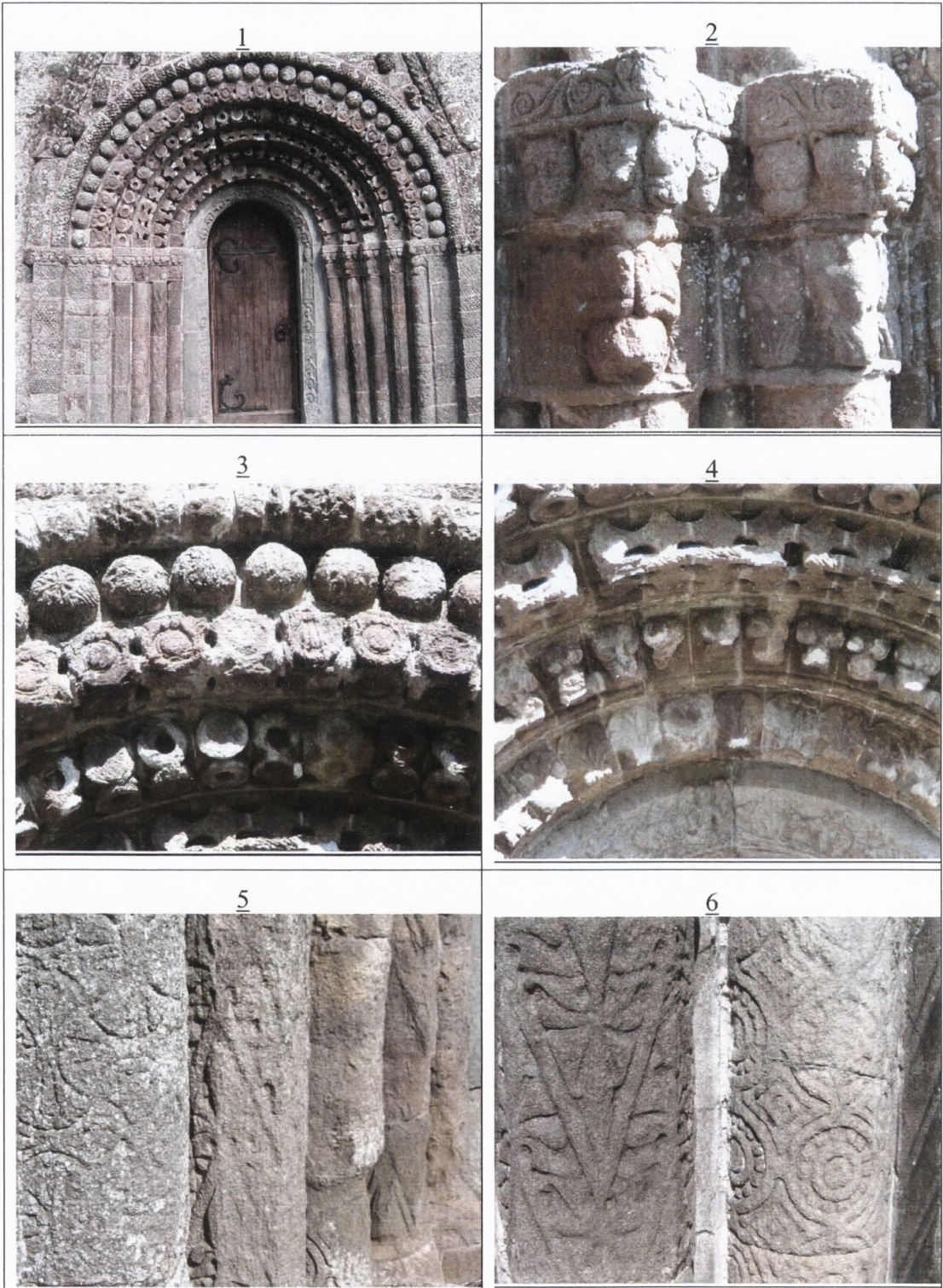
Figure 4-2: Weathering at west doorway of St. Brendan's Cathedral, Clonfert
