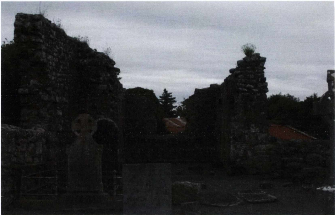
Figure 5.17 Annaghdown priory, Galway: view of the east end of the church with all tracery removed
