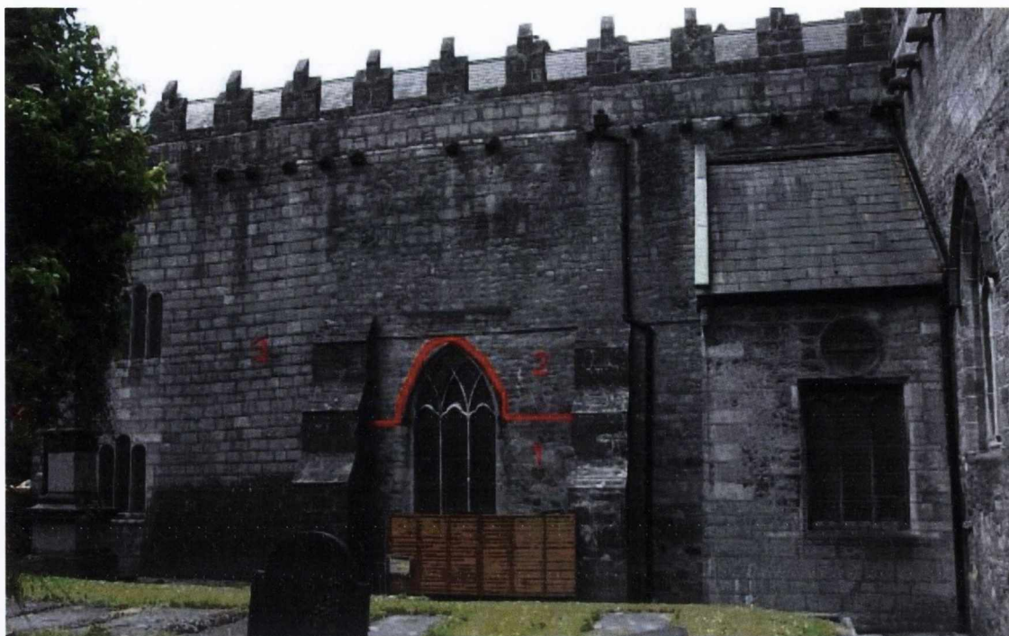
Figure 5.9 St. Nicholas collegiate church: south transept external east façade with masonry phases after Jim McKeon
