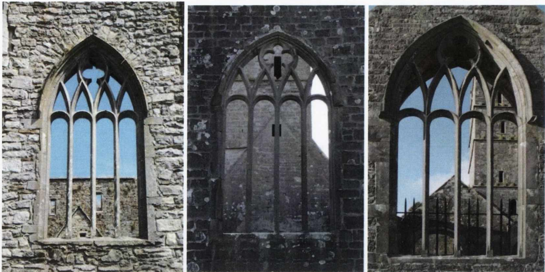
Figure 7.12 Nave west, Cashel Dominican friary (left) and chancel east (middle) and south transept south (right), Moyne Franciscan friary
