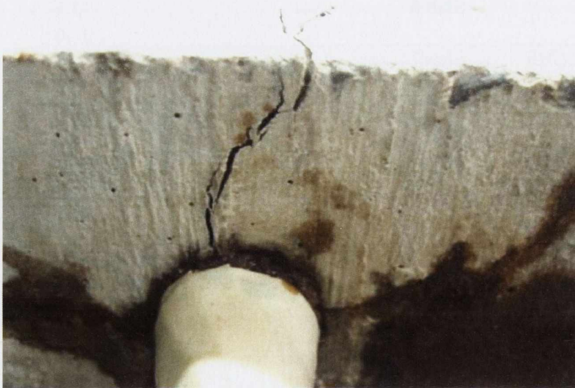
Figure 5.14. Propagation of cracks in three directions away from the reinforcing bar
