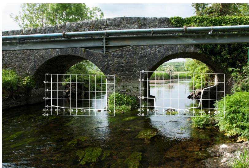
Figure 4.6: Upstream view on the Fergus River at Crossard Bridge at low flow. The diver is installed at the left bottom of the right arch.
