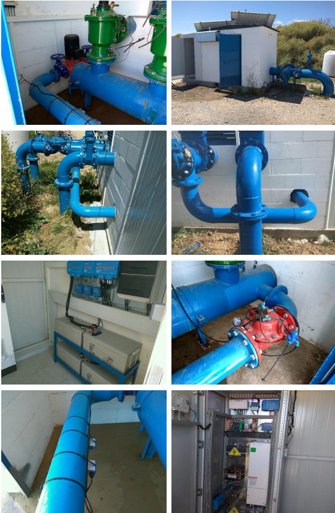
Figure 7-7. Different views of the MHP plant, showing the PAT, PRV, bypass connection, monitoring system (flow meter) and regulation chart.
