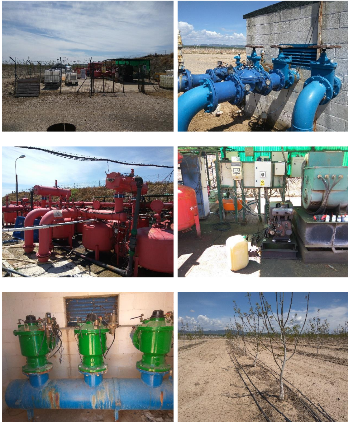
Figure 7-3. Aerial view of the reservoir feeding the irrigation networks and different views of the farm prior the PAT installation. a) Reservoir that feeds the irrigation network; b) Operating, storage and maintenance area; c) PRVs at the output of the hydrant; d) Filtering system located within the operating area; e) Diesel generator used at the farm; f) valves composing the hydrants inside of the concrete chamber; g) walnuts irrigated downstream of the hydrant.
