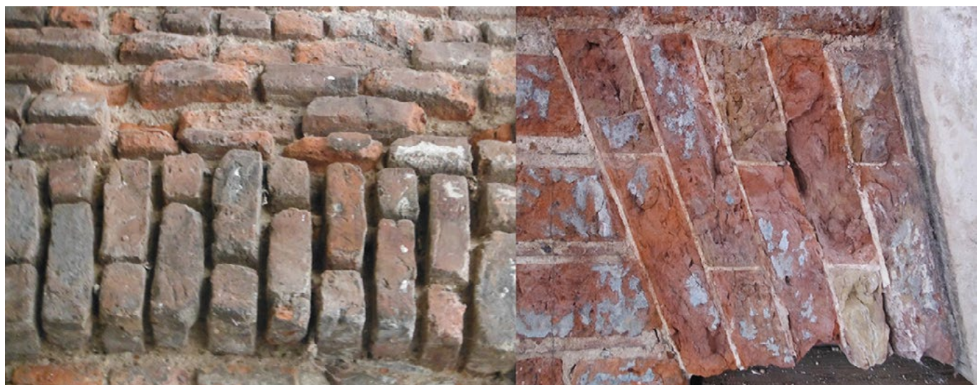
Figure 3 Comparison of the fabric of the window heads in the back wall (left) and the façade (right). Photographs by Sara Pavia.
